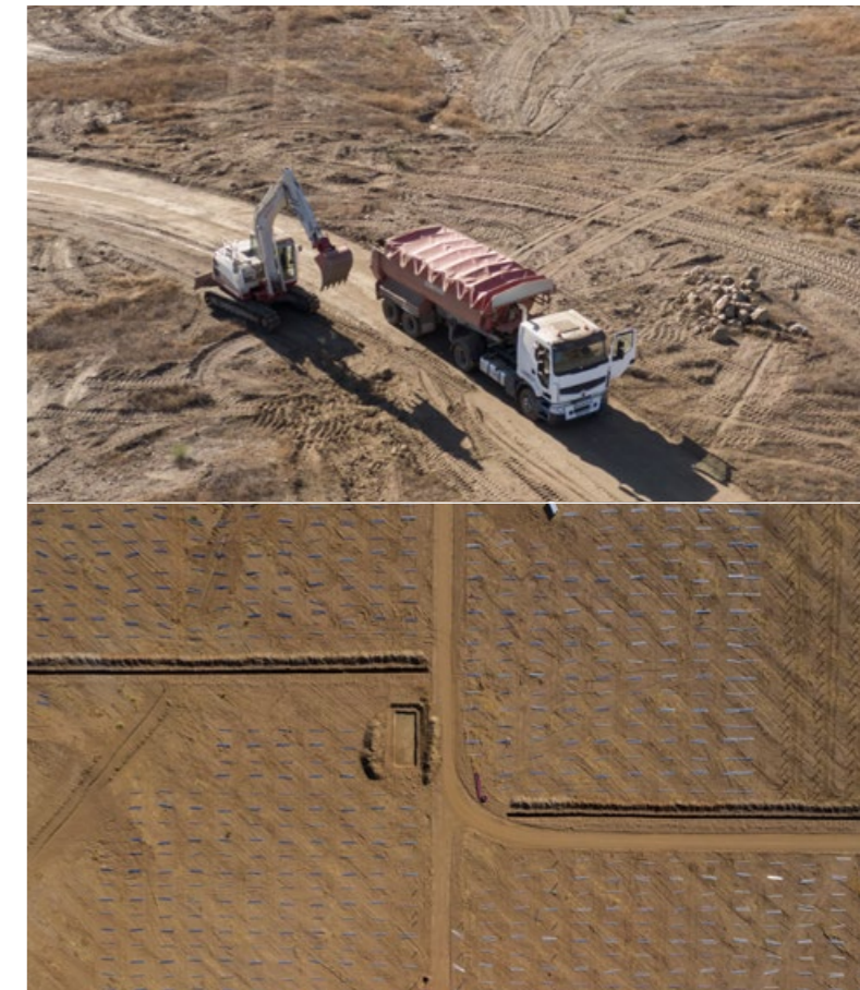
Start of construction works (September 2020) and mechanical installation works (October 2020) of La Cabrita solar PV park in Tabernas
