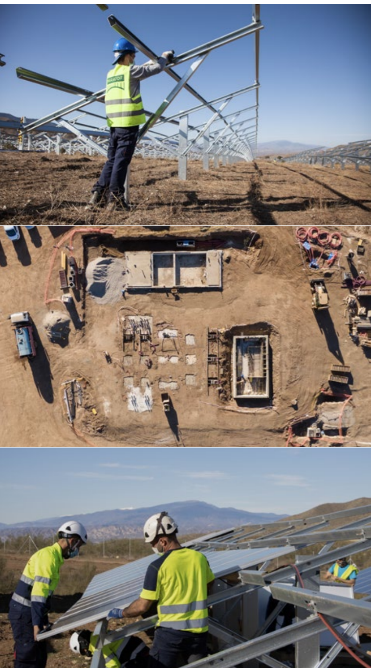
Top picture: Assembly of the mounting structure of the photovoltaic modules at La Cabrita solar park Middle: Construction of the substation Bottom picture: Installation of the modules
